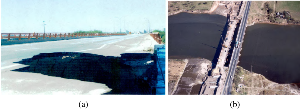
Figure B.3: Bridges of the Santa Fe-Rosario Highway over the Salado River during and after the 2003 flood. (a) Collapse of the westward abutment; (b) Reconstruction after the flood.
