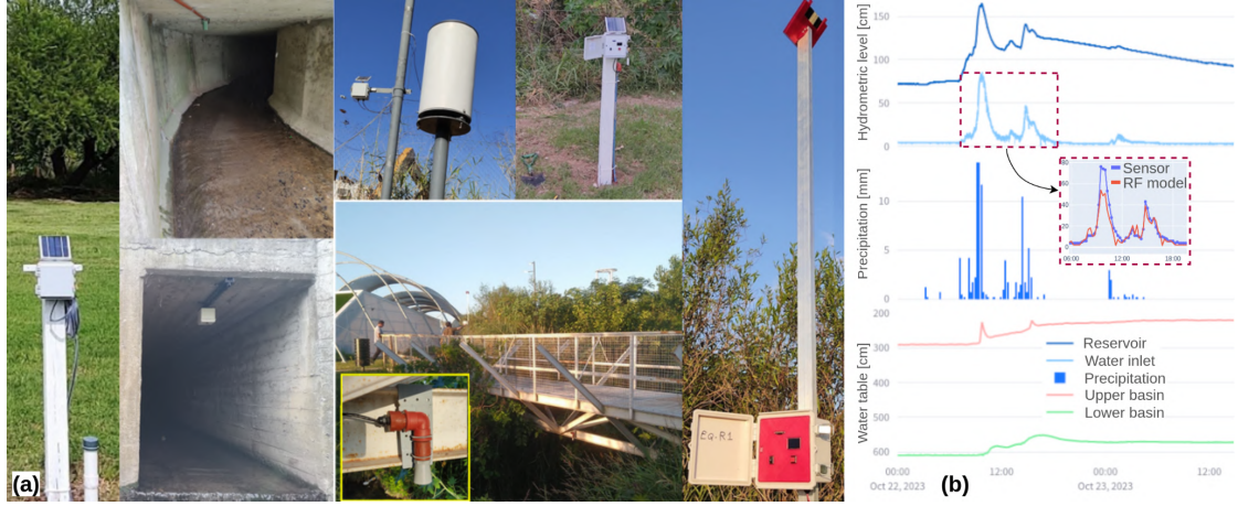
Figure A.7: (a): Instrumentation of the WUNR (see aerial view in Figure A.6(b)) at various points along the urban catchment. The outlet of the main drainage channel is also shown. (b): from top to bottom, the temporal evolution of the water level at the reservoir, at the drainage outlet, the precipitation and the groundwater level in the urban catchment and at the entrance to the reservoir. The inset shows the water level predicted by the random forest model.
